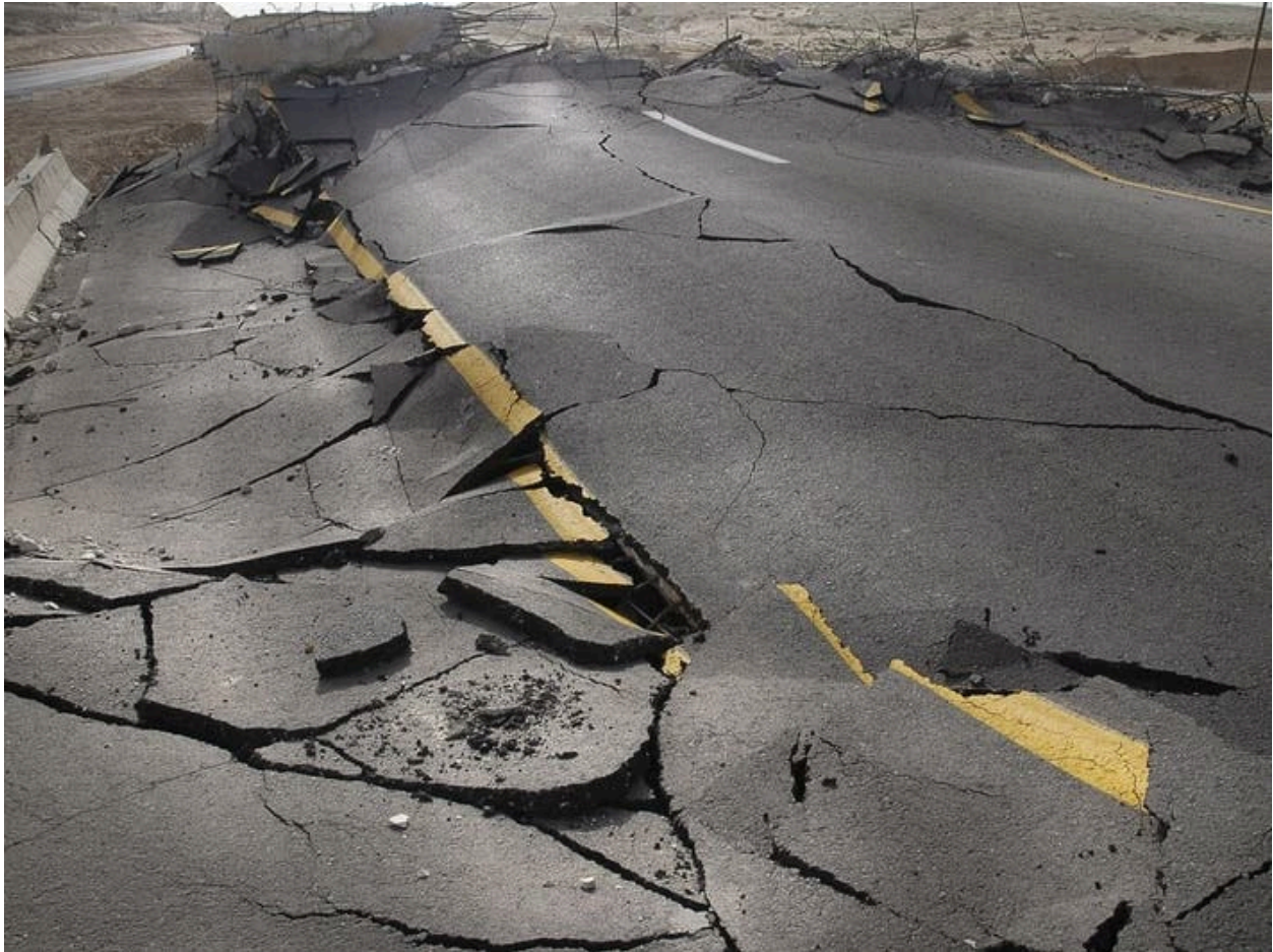
Highway destroyed by Ridgecrest Earthquake. Source: Shutterstock
