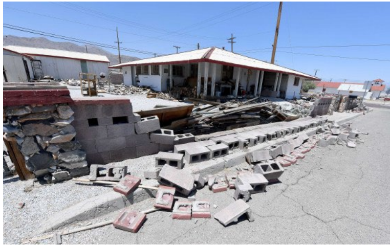
A cinder block wall collapsed onto the street outside a home in Trona. Source: Will Lester, Inland Valley Daily Bulletin/SCNG
