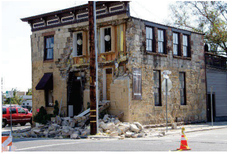
Figure 4. Image of damaged two-story building.
